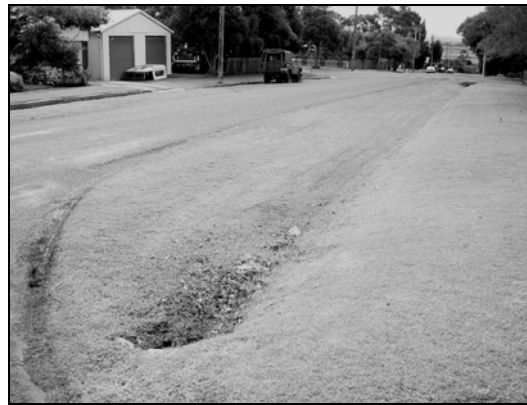
Grassed swale drain in a minor street of Morpeth
