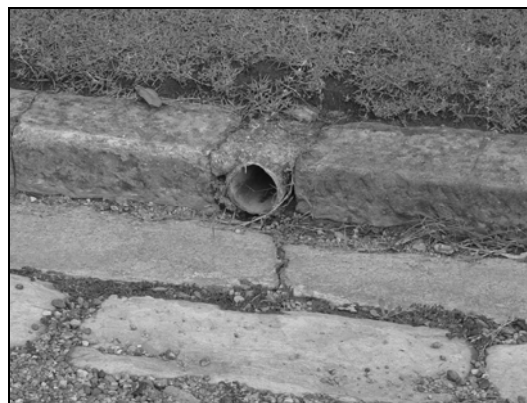
Residential stormwater outlet utilising an existing hole within the kerb and guttering.
