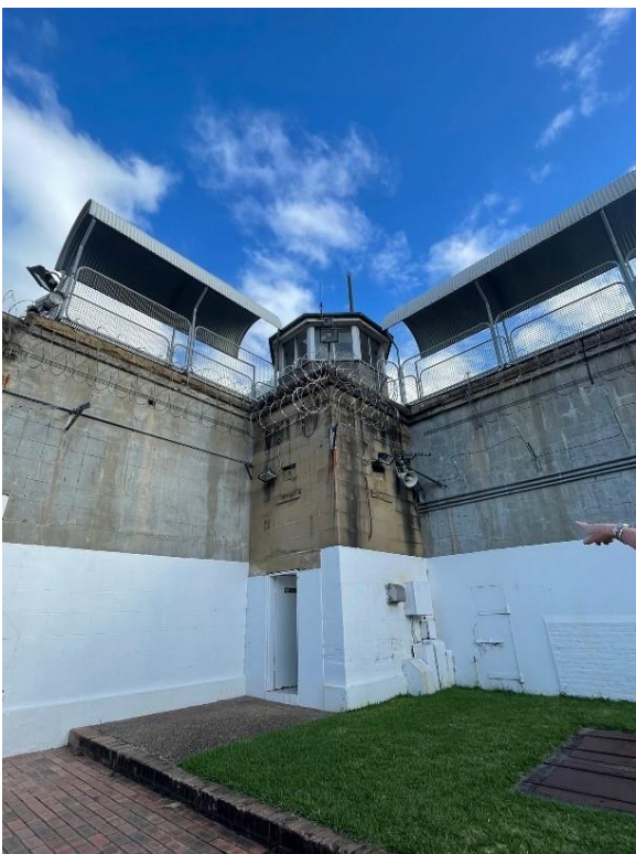
Figure 2 - Existing Tower 1 where stairs are to be installed for tour entry. Existing doorway opening to be maintained.
