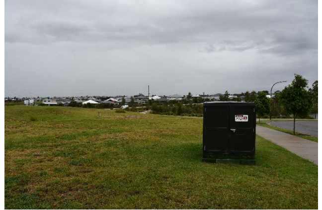
Figure 11 Electricity services along Suncroft Street
