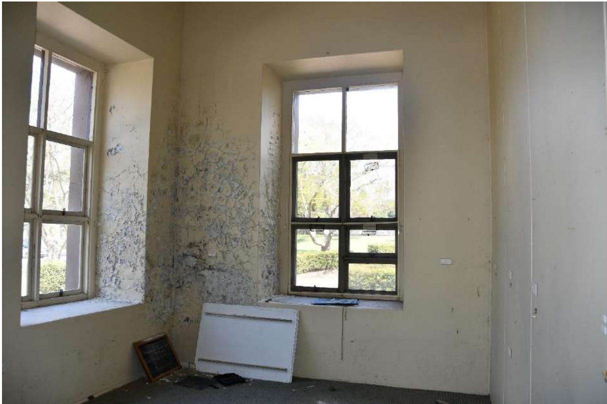
Figure 44: The Office (Room #02) in Main Pumphouse (A) demonstrating water damage. Cracks in the render are visible on the external wall.
