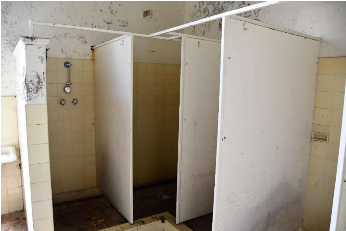
Figure 69: Showers within the northern room of the Eastern Annex showing flaked paint and tiled walls.
