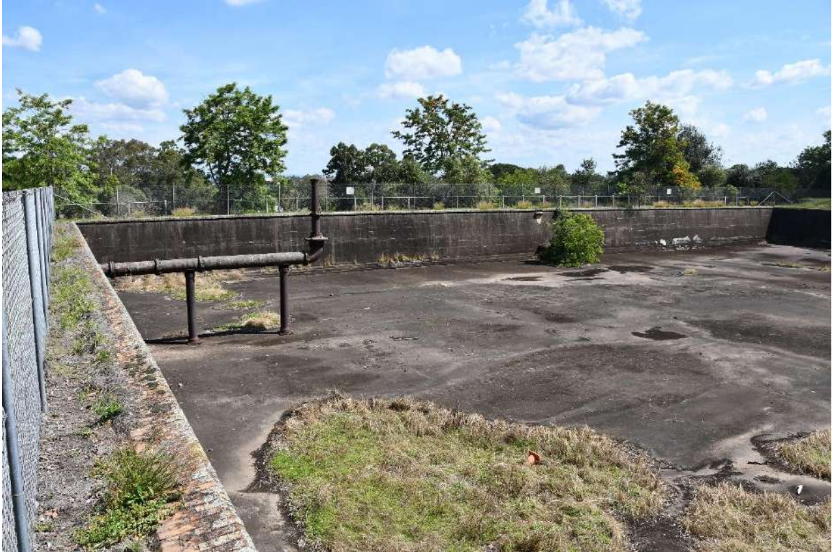
Figure 96: The Settling Tank. The inlet from the eastern wall is clearly visible. Outlets on the southern wall are obscured by trees. Cracking on the wall render is evident as well as the linear marks on the floor. View to the southwest.
