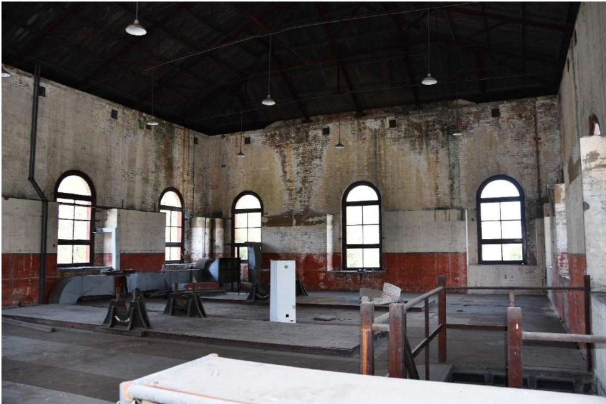
Figure 52: General view of the upper floor. Showing the original painted water damaged walls, floor and wheel brackets in place. Various later vents and ducting are additionally visible.
