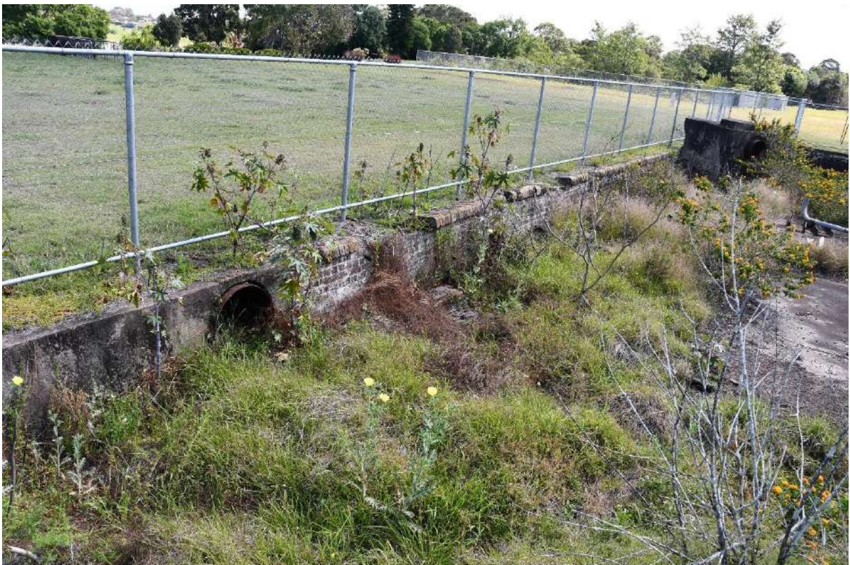
Figure 100: The southern wall of Filter Bed 2 (Item I-2) where the concrete modifications from the 1950s adaptations, are clearly visible. View to the southeast
