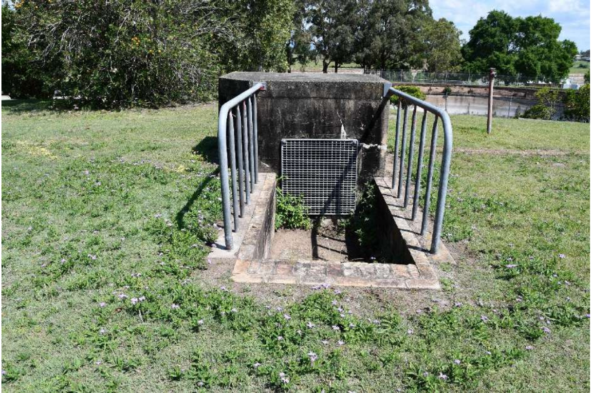
Figure 41: Example of above ground pipe access (N)
